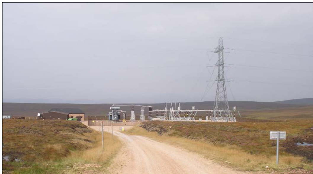
Plate 4.3: Existing Gordonbush Wind Farm Substation
